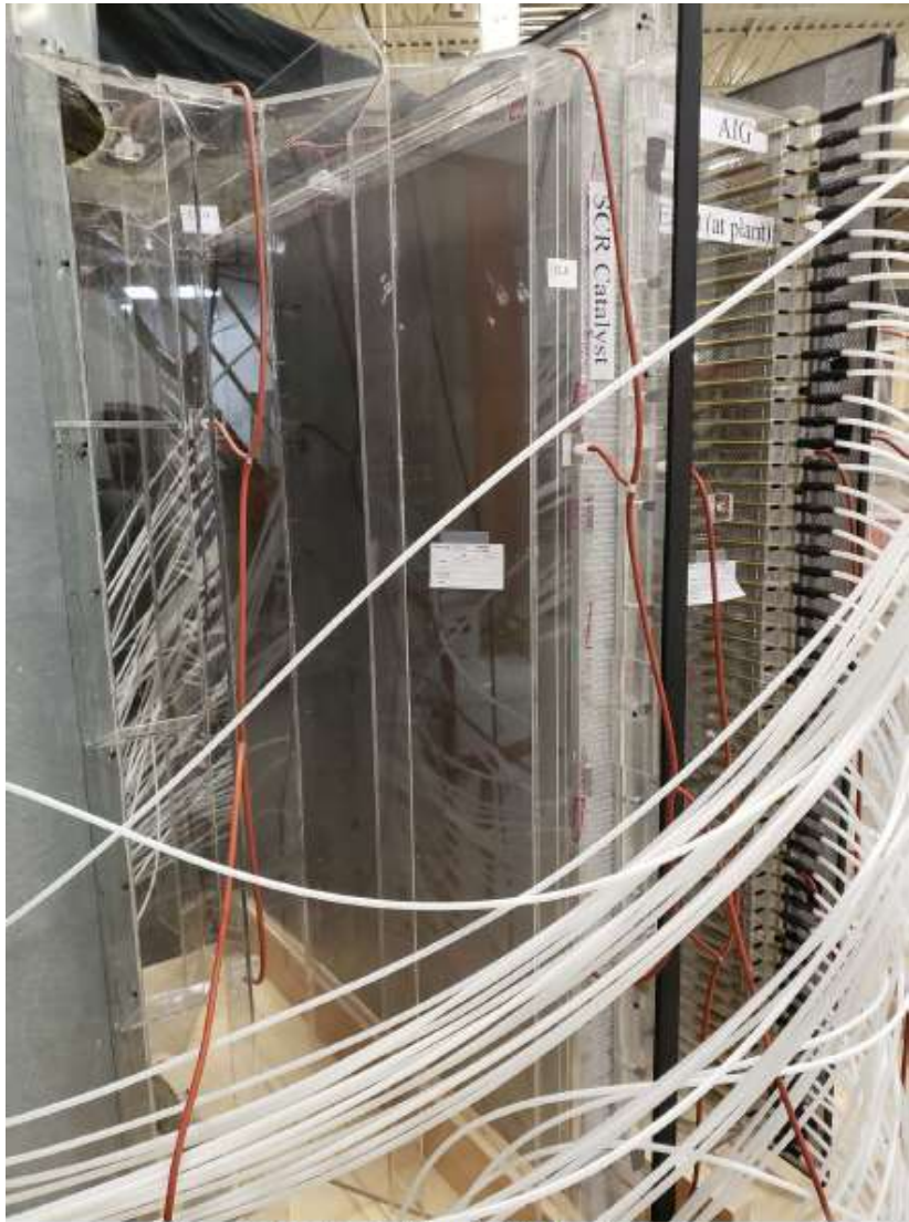
SCR Catalyst - View Looking Northwest
