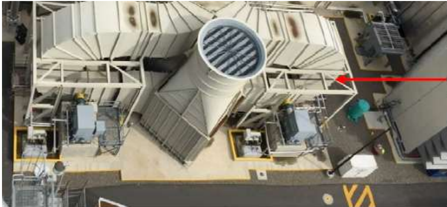
Tempering Air Fans
